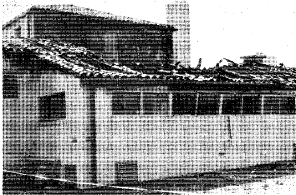
Kitchen damage visibly seen from outside of Officers Club.
